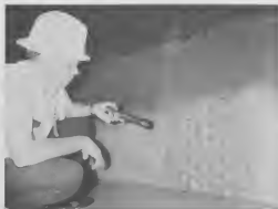
Franklin Dowling of Mechanical Engineering Division inspects a riveted section where special care is needed in applying the fiberglass coating.
